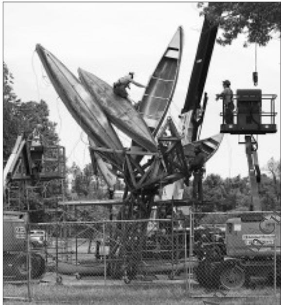
A large sculpture by Nancy Rubins is assembled on the lawn in front of Albright-Knox Art Gallery. The work, which measures about 60 feet wide and 40 feet high, will use steel cables to connect a collection of aluminum boats.
